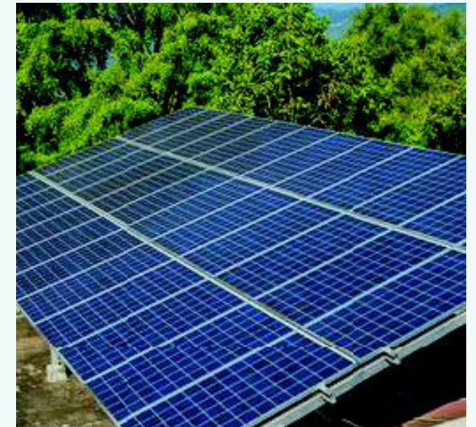
Fig 5. Roof covered in solar panels
