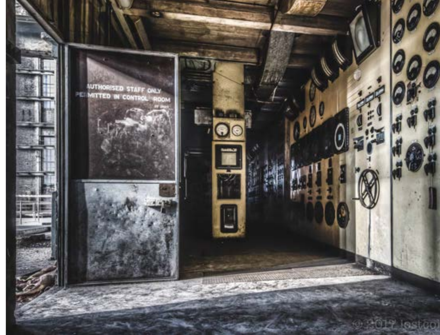
Lost Collective image a Control Room at WBPS (Patman, B. 2015).
