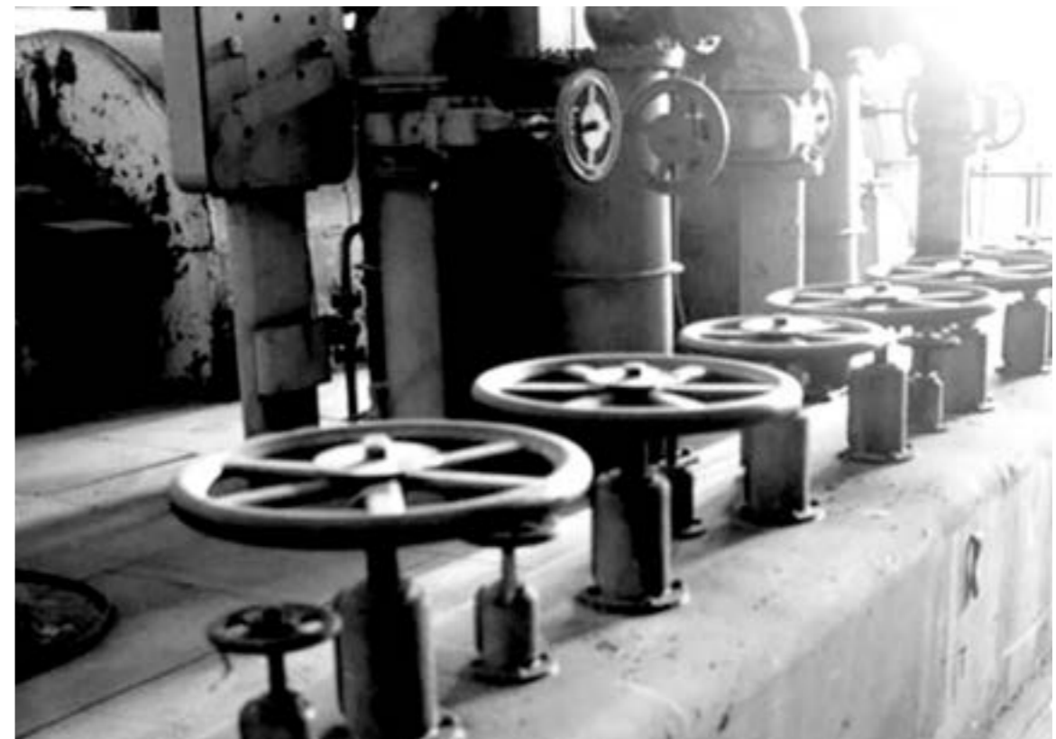
Parsons turbine and pumps, WBPS.
