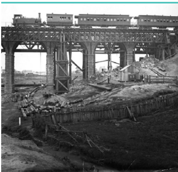
Upgrade of rail bridge at Lewisham, 1886 (Source: Australian Railway Historical Society NSW)
