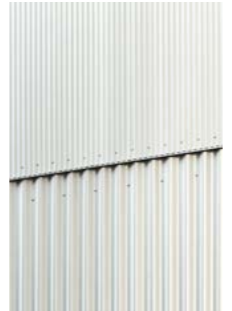
2 Varying scales of metal cladding profiles (Maggie Street Curious Practice. Image Alex McIntyre)
