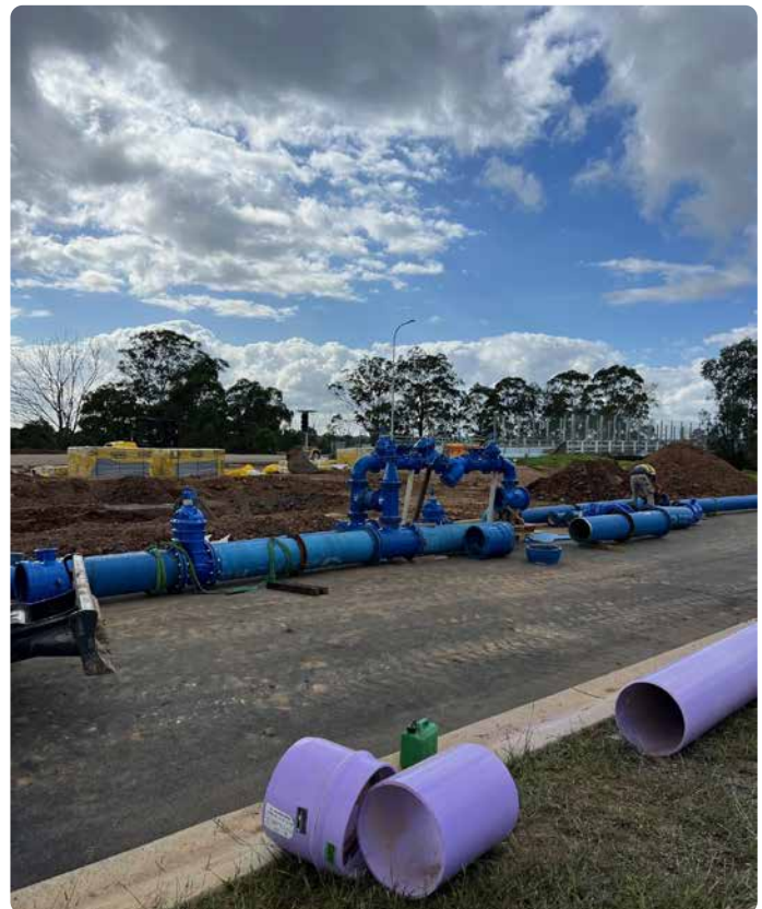
Purple pipes being laid for recycled water supply at Panorama, North Wilton
