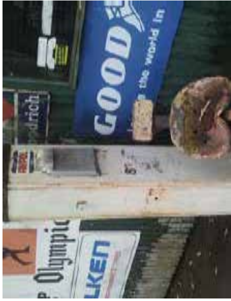
Photograph 21: Parcel 6 bowser that was not connected
