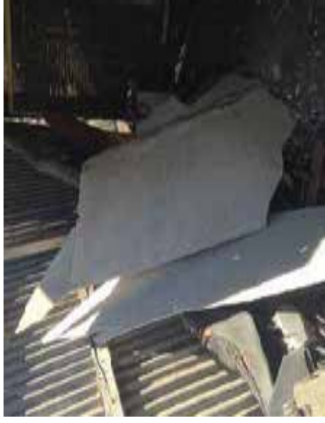
Photograph 66: Potential ACM present within the shed in Parcel 14
