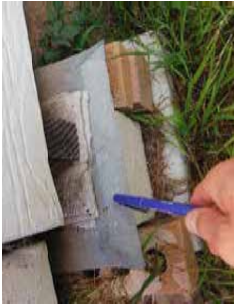
Photograph 73: Potential ACM on Parcel 16
