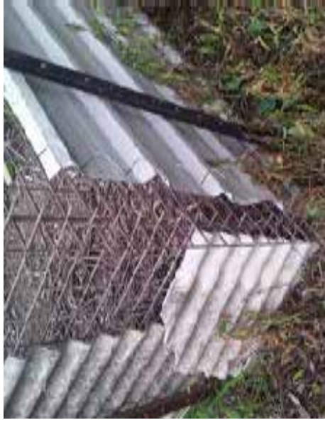
Photograph 33: Parcel 6 ACM sheeting used as fence along chicken coup
