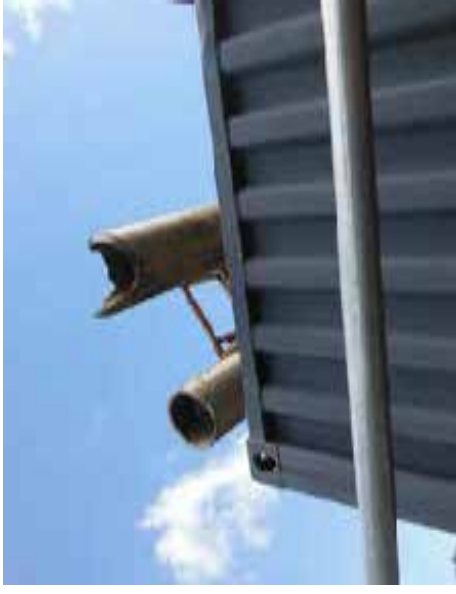
Photograph 213: Potential ACM pipes on Parcel 88
