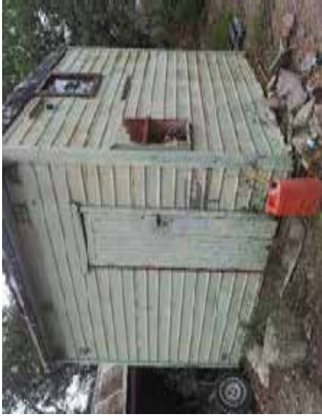
Photograph 9: Parcel 5 corrugated metal shed, with paint flaking
