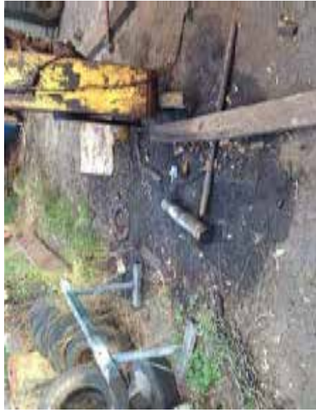
Photograph 94: Soil staining in Parcel 22
