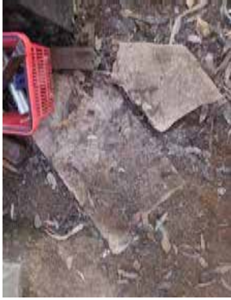
Photograph 146: ACM present adjacent to shed on Parcel 37
