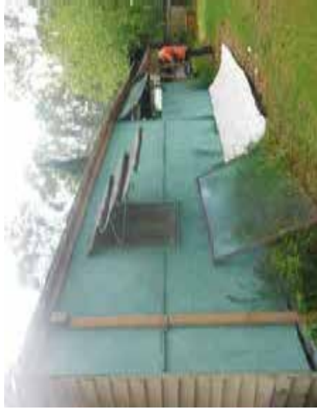
Photograph 71: Potential ACM contained property on Parcel 16
