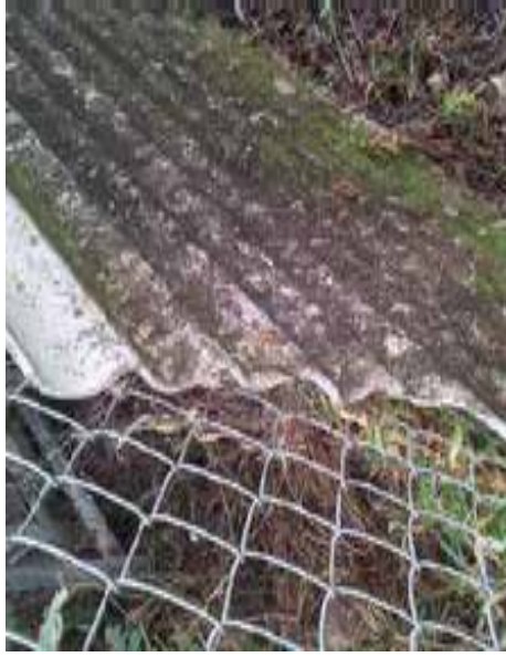
Photograph 32: Parcel 6 ACM sheeting used as fence along boundary
