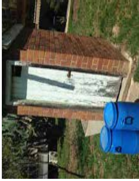
Photograph 180: Parcel 50 potential septic tank
