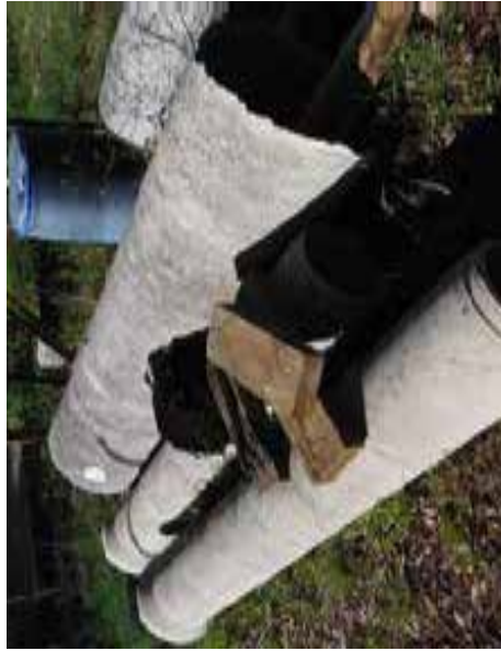
Photograph 196: Potential ACM pipes on Parcel 55
