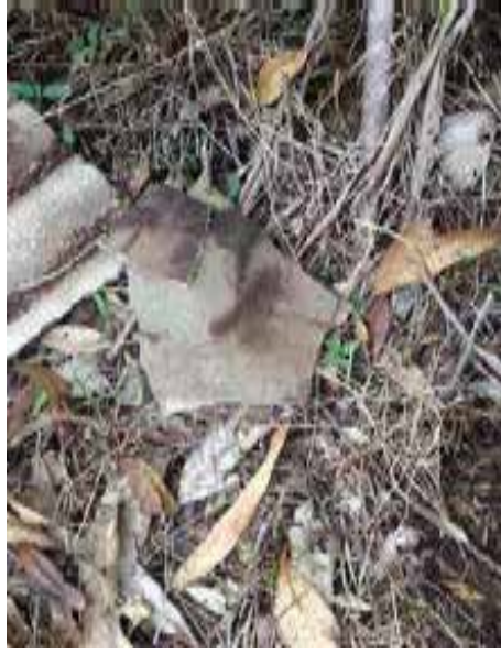
Photograph 83: ACM at surface within Parcel 19
